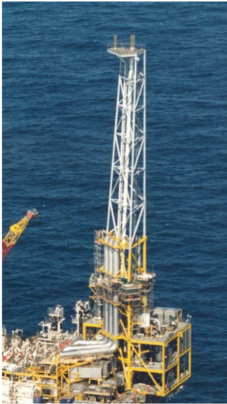
Offshore application for production flare
