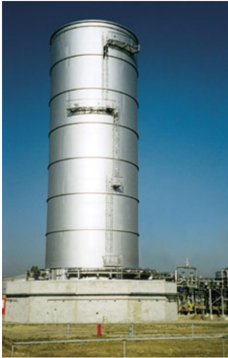
Totally Enclosed Ground Flare
