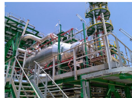
Heaters for Stabilizer column
