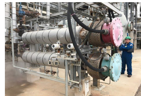
Regen Heaters for Alkyllation, Chevron El Segundo, CA
