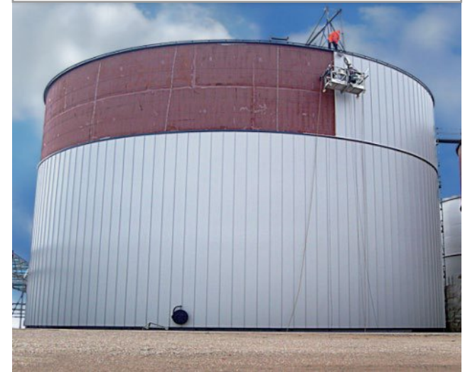
Large tank insulation (TracLoc)
