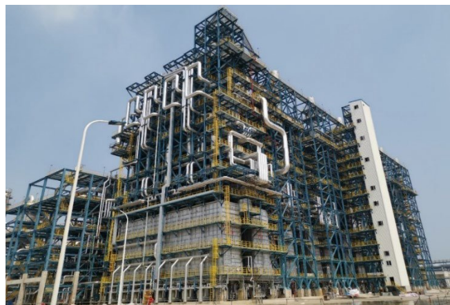
Zhongke 800 KTA Ethylene Complex (World's Largest Gas Furnace)
