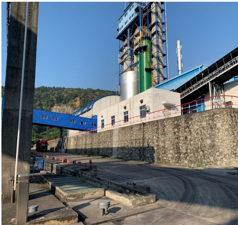
No. 3 Coking Unit for Guangdong Petrochemical Company
