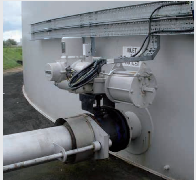
Figure 2: Triple excentric butterfly valve ZWICK TRI-CON used as ESD-Valve on a storage tank in Scotland
