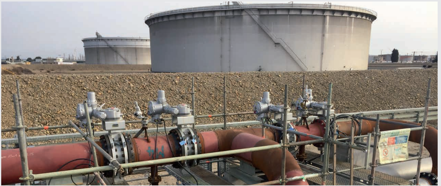
Figure 3: Tankstorage pipeline system with TRI-CON butterfly valves
