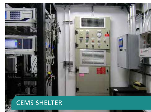
EXTRACTIVE OXYGEN SYSTEM PANEL
