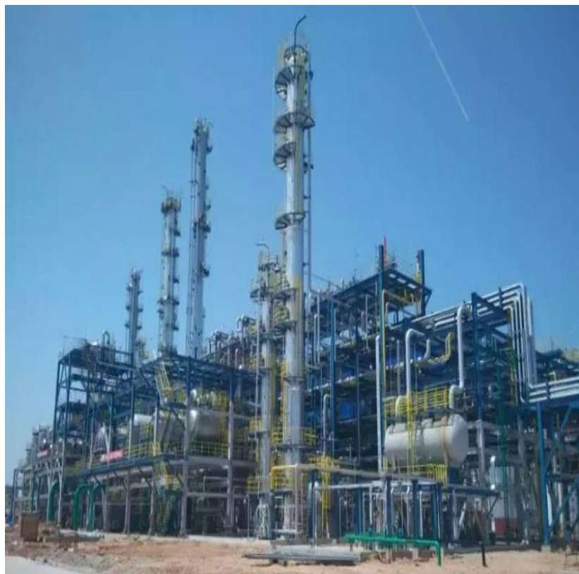
230 kta COAT™ Unit in FREP, Fujian
