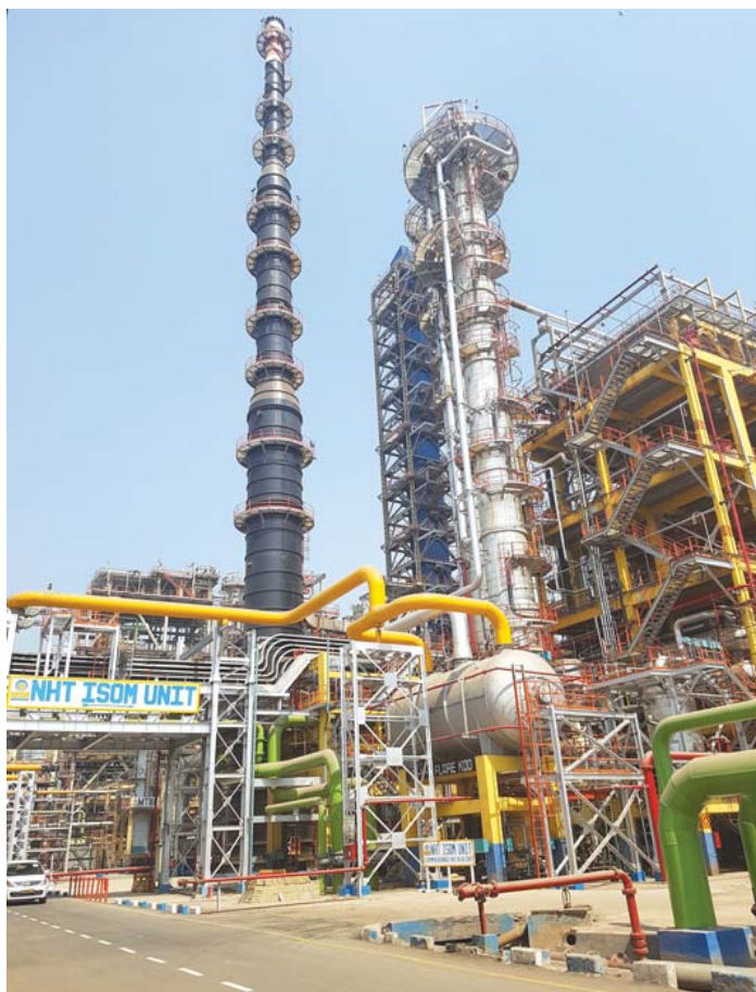
Pictured: In February 2017, Isomalk-2 isomerization unit, having capacity of 680 KTA, was commissioned at the refinery territory of Bharat Petroleum Corporation Limited (Mumbai, India) with the direct participation of SIE Neftehim, LLC experts.
