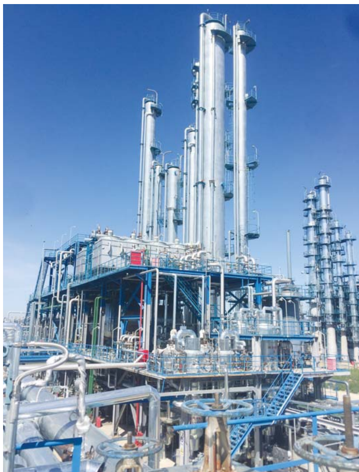
Pictured: N-butane isomerization unit using Isomalk-3 technology at Liaoning Hualu Specialty Asphalt Co, (Liaoning Province, PRC).
