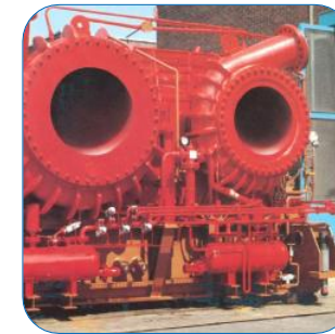
Heat pump "Rya", Delivery 1984, still in operation
