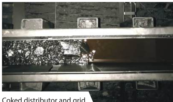
Coked distributor and grid
