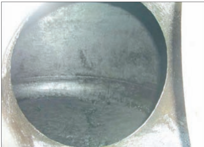
Figure 7 Online cleaning of slop distillation unit: main fractionator bottom before online cleaning
