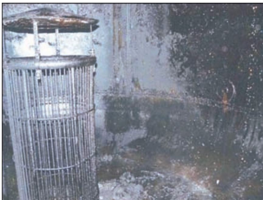
Figure 2 Visbreaker main fractionator bottom
