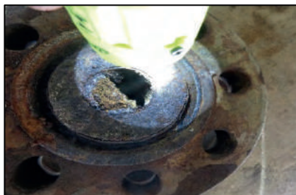
Figure 7 Inspection after shutdown showed that the outlet piping of the knockout drum was plugged
